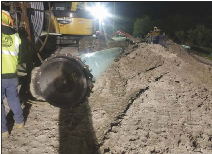
Figure 6. Tail End of Fusible Polyvinyl Chloride Pipe After Completing Pullback Under Boca Ciega Bay
